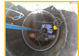
Eric W and Martin B working on the motor that draws up the surplus rainwater from our underground tanks - a protracted issue that we think has been finally fixed.
